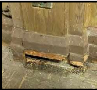
Figure 68: Baseboard exhibits termite damage.
