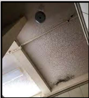
Figure 72: Popcorn ceiling shows mold from water damage.
