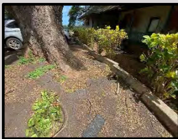
Figure 84: Tree roots breach through the asphalt pavement. Source: FAI Architects, 2023
