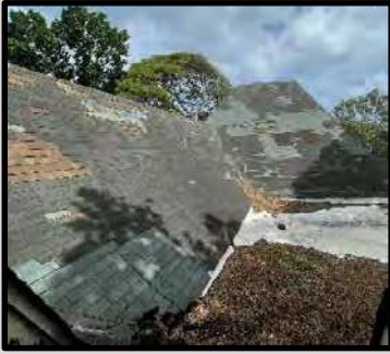
Figure 73: Roof exhibits sagging and damaged asphalt shingles from water damage. Source: FAI Architects, 2023
