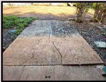
Figure 82 : Uneven surface Source: FAI Architects, 2023
