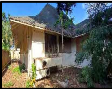
Figure 75: Roof exhibits structural damage.
