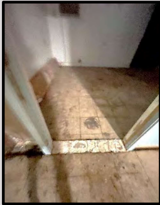
Figure 79: Water damage to VCT tile flooring. Source: FAI Architects, 2023
