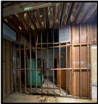
Figure 71: Wood stud framing wall with water damage.
