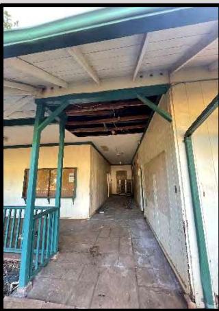
Figure 74: Supporting wood members exhibits water damage. Source: FAI Architects, 2023
