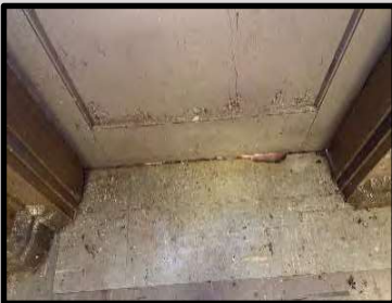
Figure 80: Termite damage to interior door. Source: FAI Architects, 2023
