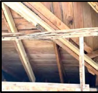
Figure 67: Ceiling studs displays termite damage.
