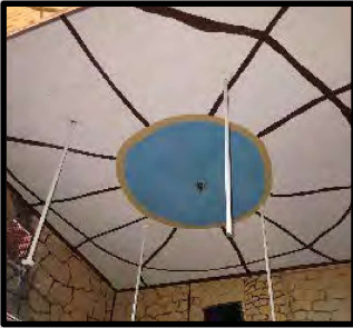
Figure 70: Exposed electrical wires in the FCU office.
