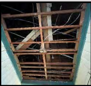
Figure 69: Exposed electrical wires of main entrance ceiling.
