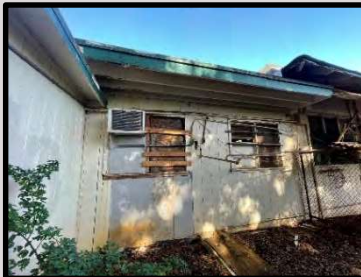
Figure 78: Deterioration of exterior wood siding.
